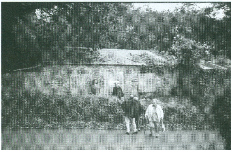
The miners' cottages as they face the road. The lower cottage juts out beyond the upper one. The central door and windows of the upper cottage are here boarded up awaiting essential consolidation work on lintels. 22/6/02
