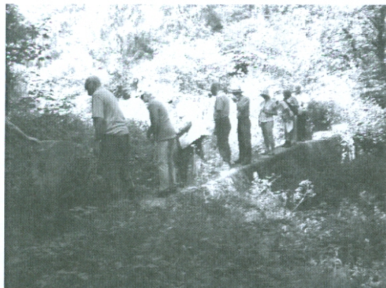
Members inspecting the dam with its sluice gate on the right. They are looking upstream towards the reservoir, now largely overgrown with water-loving plants
