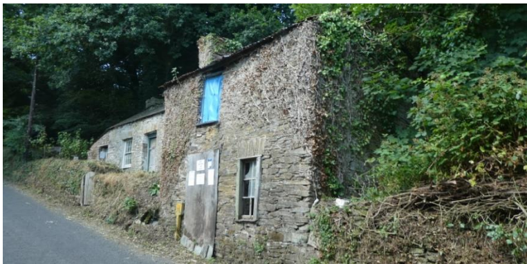
The miners' cottages from the south, looking uphill from Luckett, 14 July 2018. See item above concerning the renovation of the lower door
