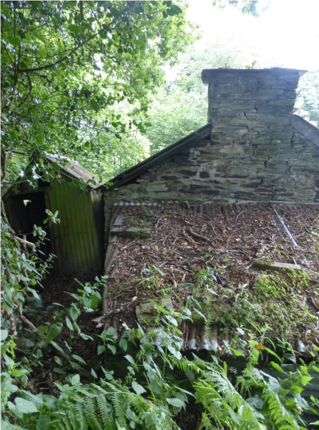
The outside W.C. parting from the back wall of the cottages, July 2012.
