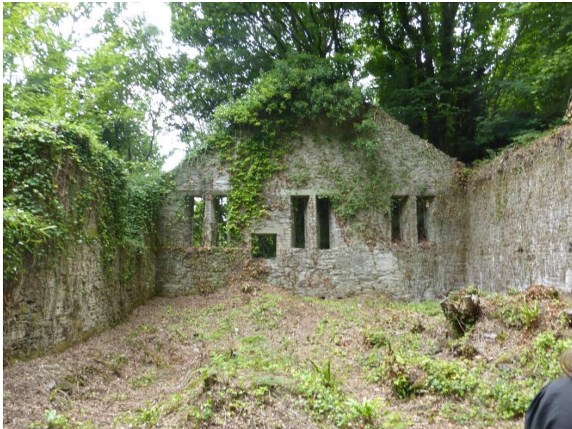
The jigger house with distinctive slit windows. After the crusher, the ore was taken to the jigger house where the task of separating the heavier ore from the lighter waste rock began.
